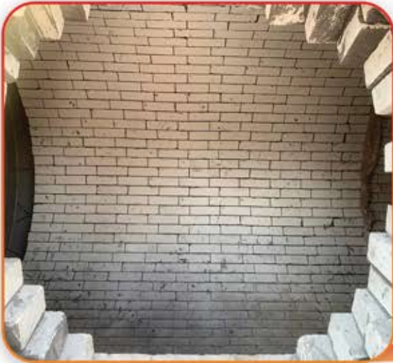
○ Rotary cement kiln
